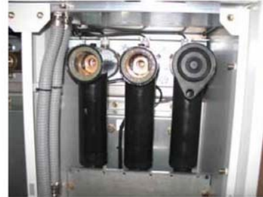
Factory mounted T-connectors Interface C with cables connected to VT's
