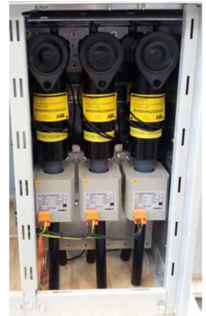
Factory mounted CT's for tariff metering
