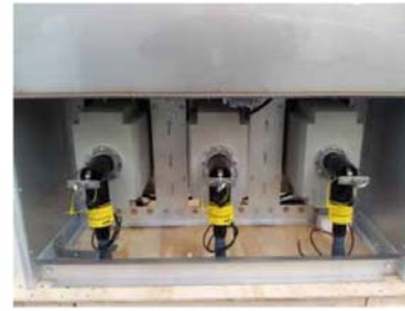
Touch proof VT's with integrated bushings (Interface A) placed in the lower back of the unit, with cables connected to the T-connectors in the cable compartment in front
