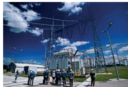
Siedlce Ujrzanow substation (© PSE SA)
