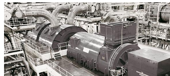
Power Plants and Turbines
