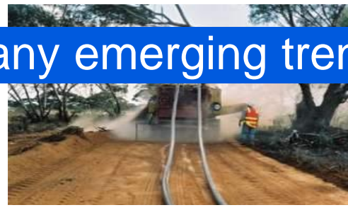
Murraylink, Australia, world's longest underground cable
