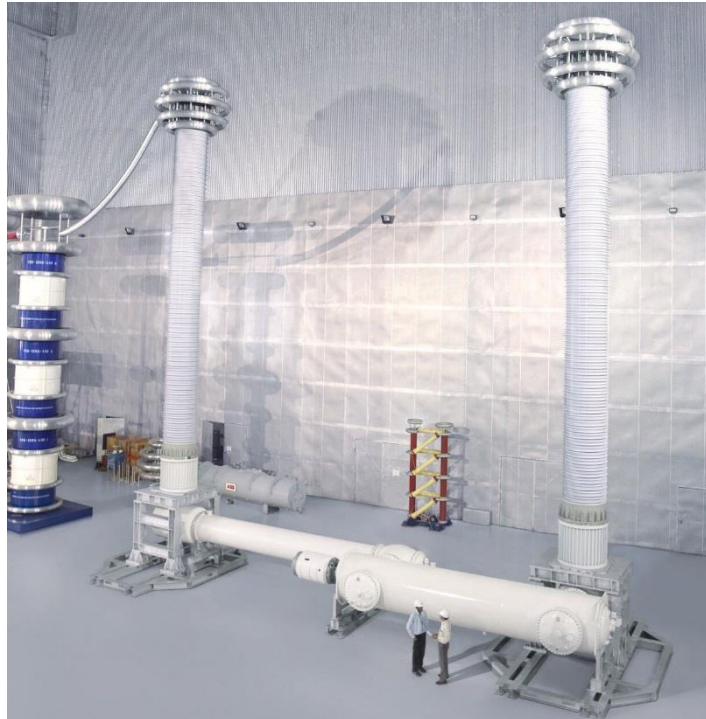
1,200 kV AC circuit breaker, transformer
