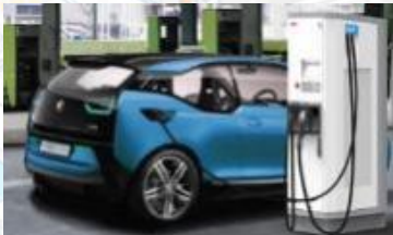
EV charging with cloud management
