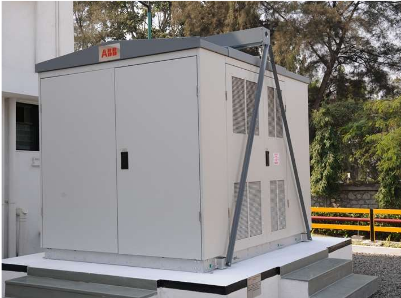
Compact Secondary Substation- 11kV
