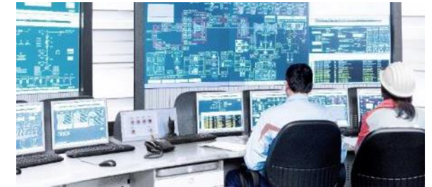
SCADA automation, RTU, AI/ML for jetty pipeline
