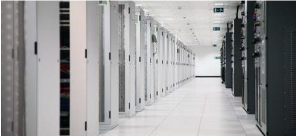
Power distribution solutions for data center major and IT majors
