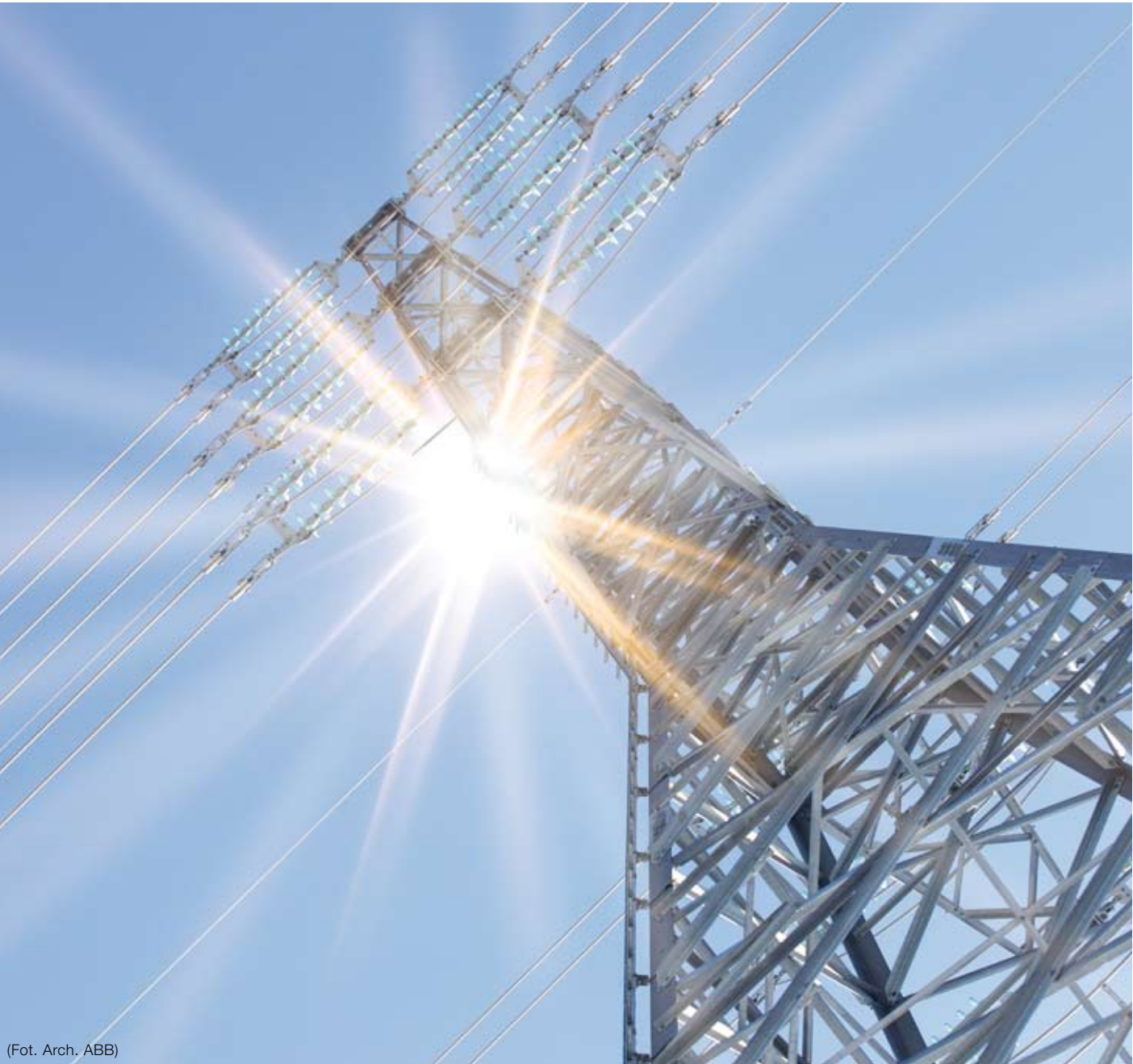
(Fot. Arch. ABB)
