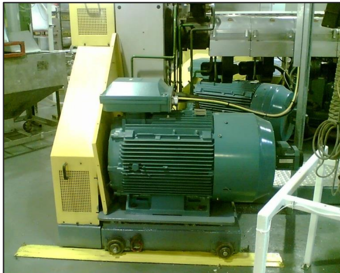
Caption: ABB drives and motors save £80,000 a year for plastic extruding company.
