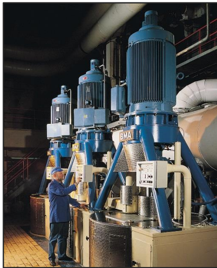
Caption: ABB multi-drives are being used to drive three centrifuge units for the spinning off of sugar crystals from solution at British Sugar Newark’s factory.
