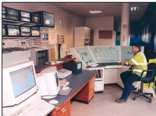
Caption: Carbon dioxide levels in the Clyde Tunnel are controlled with a new SCADA system using ABB motors and drives.
