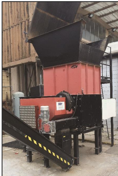
Caption: Haddonstone has avoided a £50,000 upgrade to its electrical supply by installing an ABB variable-speed drive on a wood chipping machine, know as a hogger.
