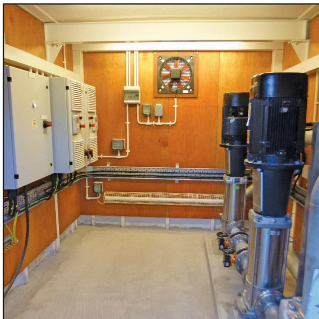
Caption: An example of Welsh Water's roadside pumping kiosk equipped with ABB variable speed drives.
