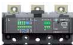
Loose trip unit
