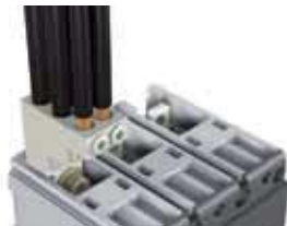
Multi-cable terminals with cables
