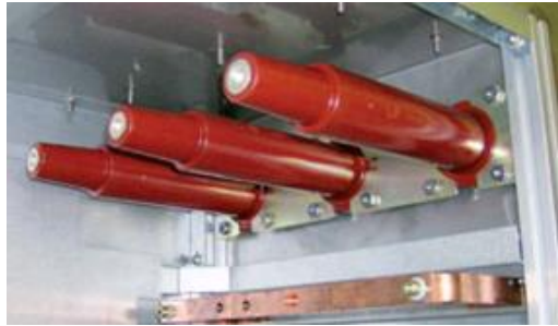
Cable termination area
