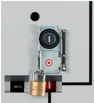
Mechanical operation for CB, with Padlock
