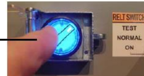
With Switch in test position REL STATUS OFF, INPUT OFF
