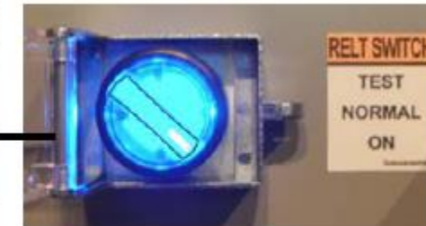
With Switch on REL STATUS ON, INPUT ON
