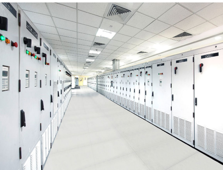
Image: Drive and PLCs feeder panel for the Compact Cold Mill for the Cold Rolling Mill Commissioning in Toronagallu, Bellary, Karnataka, India for JSW Steel Ltd.
