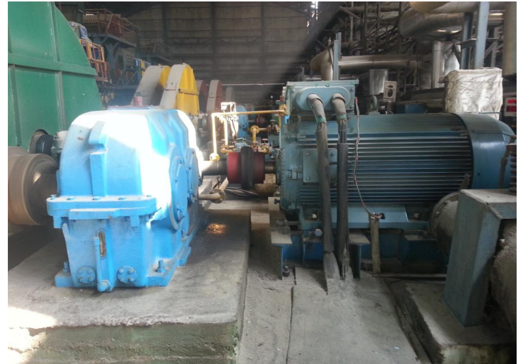
New System – Electric Motor and Drive
