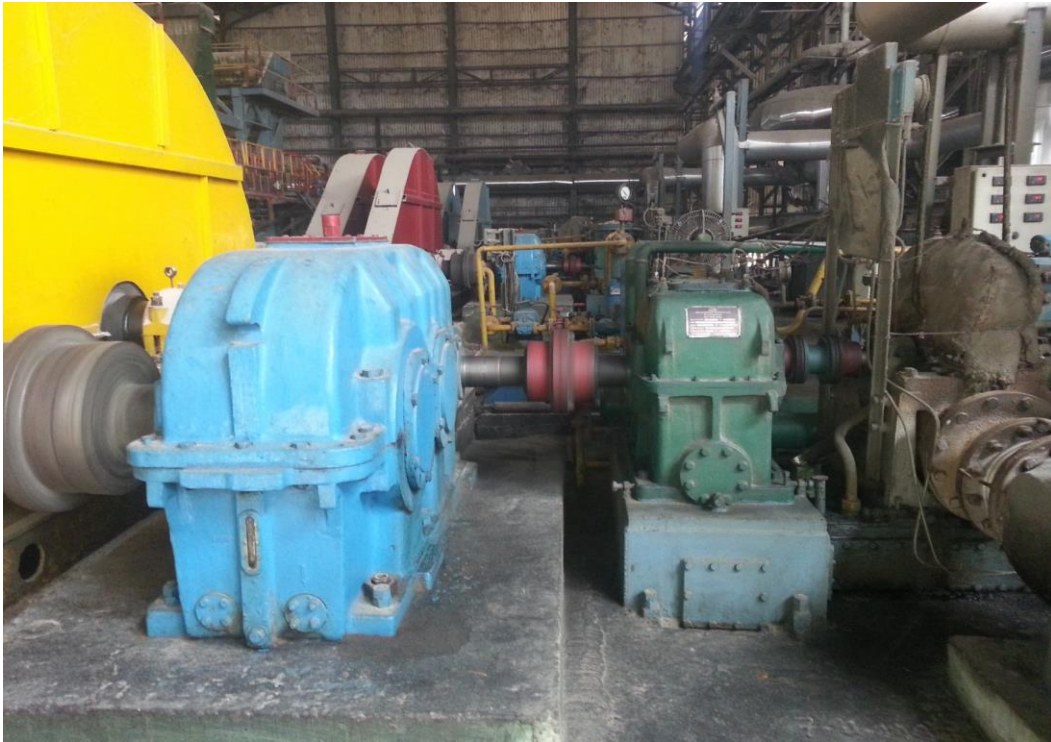
Old System – Steam Turbine
