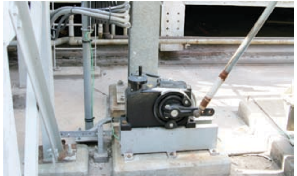
Contrac actuator on an air damper
