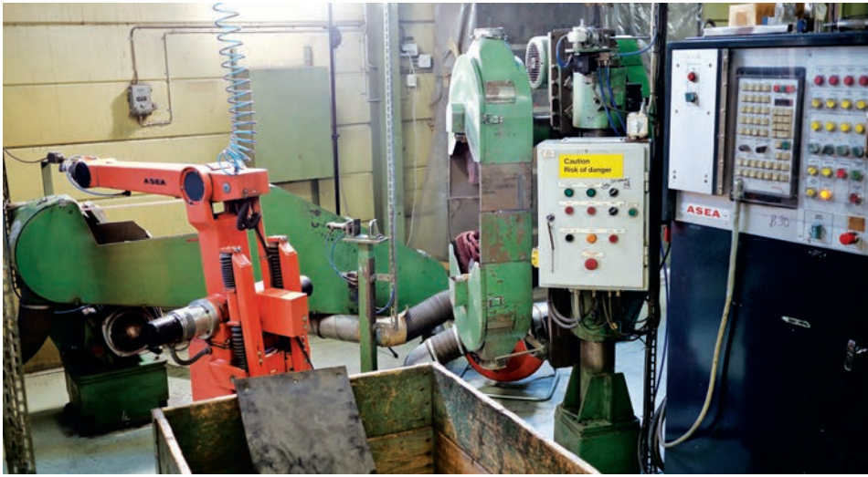
First IRB 6 customer - overview of cell
