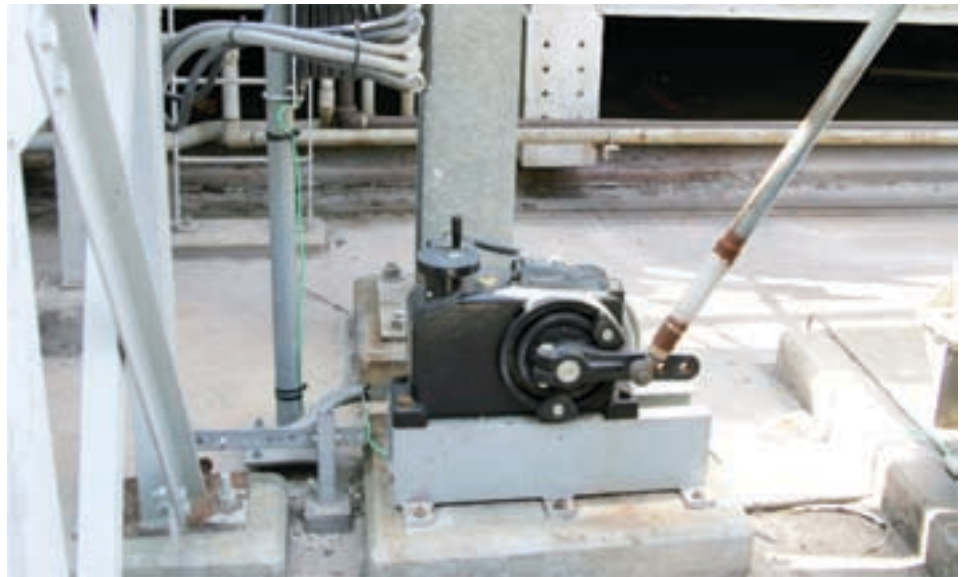
Contrac actuator on an air damper
