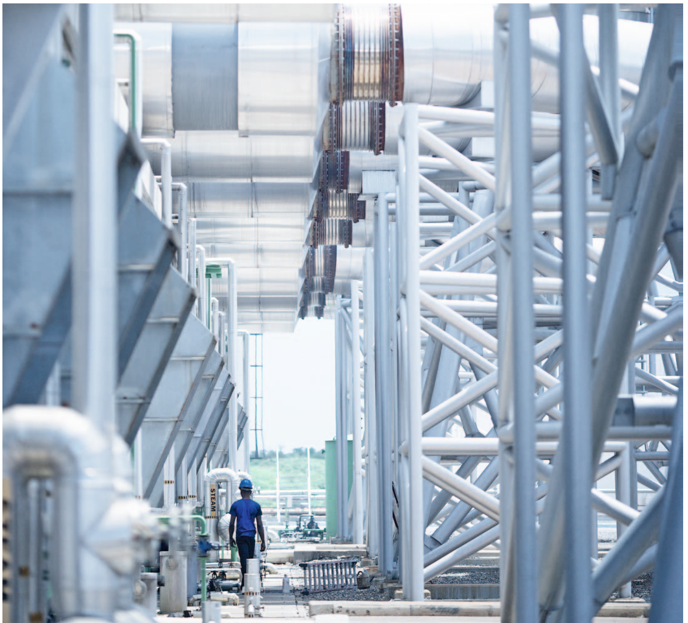
Upgraded power plant in the Dominican Republic.
