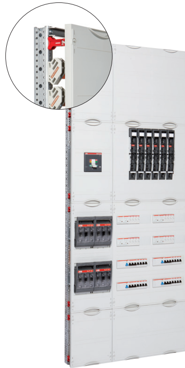
Extension with standard CombiLine N modules on WR mounting frame
